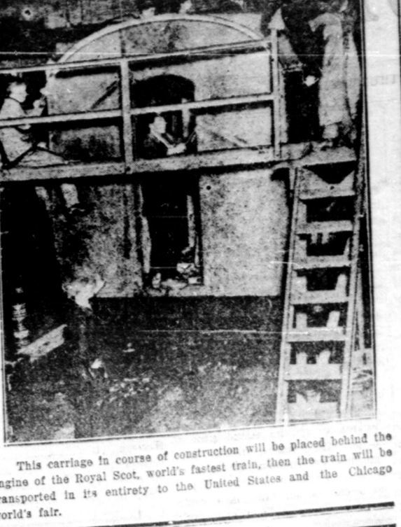
This carriage in course of construction will be placed behind the engine of the Royal Scot, world's fastest train, then the train will be transported in its entirety to the United States and the Chicago world's fair.
