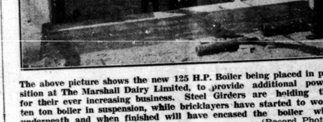
The above picture shows the new 125 H.P. Boiler being placed in position at the Marshall Dairy Limited.
