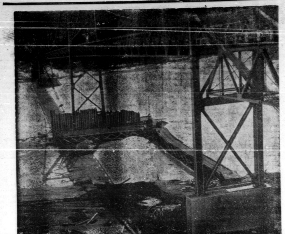
Construction Crew Saves Peace River Bridge—Pile driving starts on coffer-dam to prevent collapse of Peace River bridge, vital link in the Alaska Highway. This was opening rough-fight to prevent north pier from sinking into gravel on which it was built in wartime emergency move, rather than on abutment 15 feet further down.
