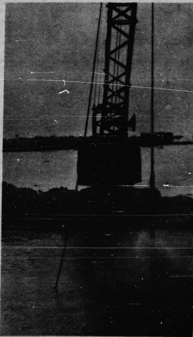
A metal ball creates a splash as workmen attempt to break rock below surface to seal a leak in a coffer dam at the $266 million Ontario Hydro site at Nanticoke.
