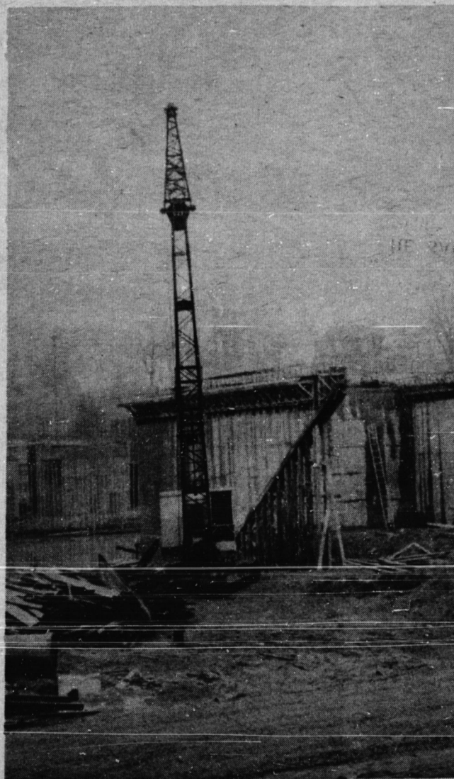
A new swing bridge is being constructed at Port Dover. The bridge will replace the old draw bridge and will permit boats to sail up the creek without interfering with traffic. (A Jim Mercer Photo)
