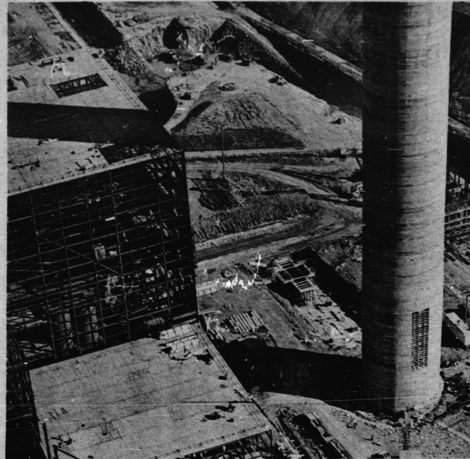
ERECTION of Structural Steel has been completed in the area of the Number 2 Boiler Bay of the Nanticoke Generating Station (high section) and the Service Bay (right). Structural Steel to the left of picture is the Turbine Hall where the 500,000 kw generator will be housed. About 25% of the total steel has been erected so far. (Ontario Hydro Photo)
