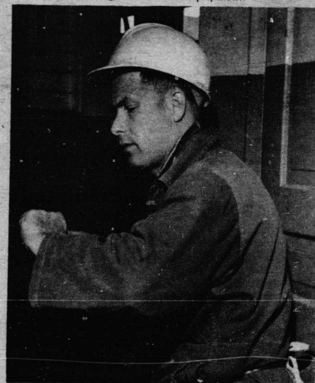
Elson Reu of Jarvis is refurbishing woodwork and putting new locks on doors in the Marshall Dairy building. (Staff Photo)
