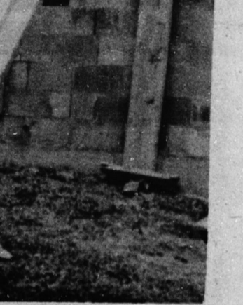
Explorer Inns Ltd. is rapidly taking shape. President Michael Lytka said the project is a month ahead of schedule because of good weather. A liquor vote is scheduled for Jan. 18 for Jarvis to determine if the new hotel will have a dining liquor lounge and a liquor lounge. (Staff Photo)
