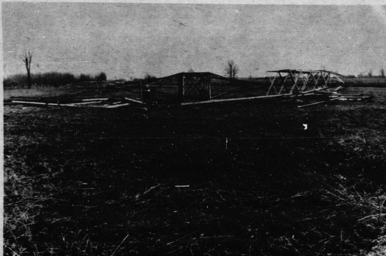
Hydro towers that will carry energy coming from the new Nanticoke Generating Station are being erected across the country side. These towers located just east of the Nanticoke Road are awaiting construction crews. (Staff Photo)
