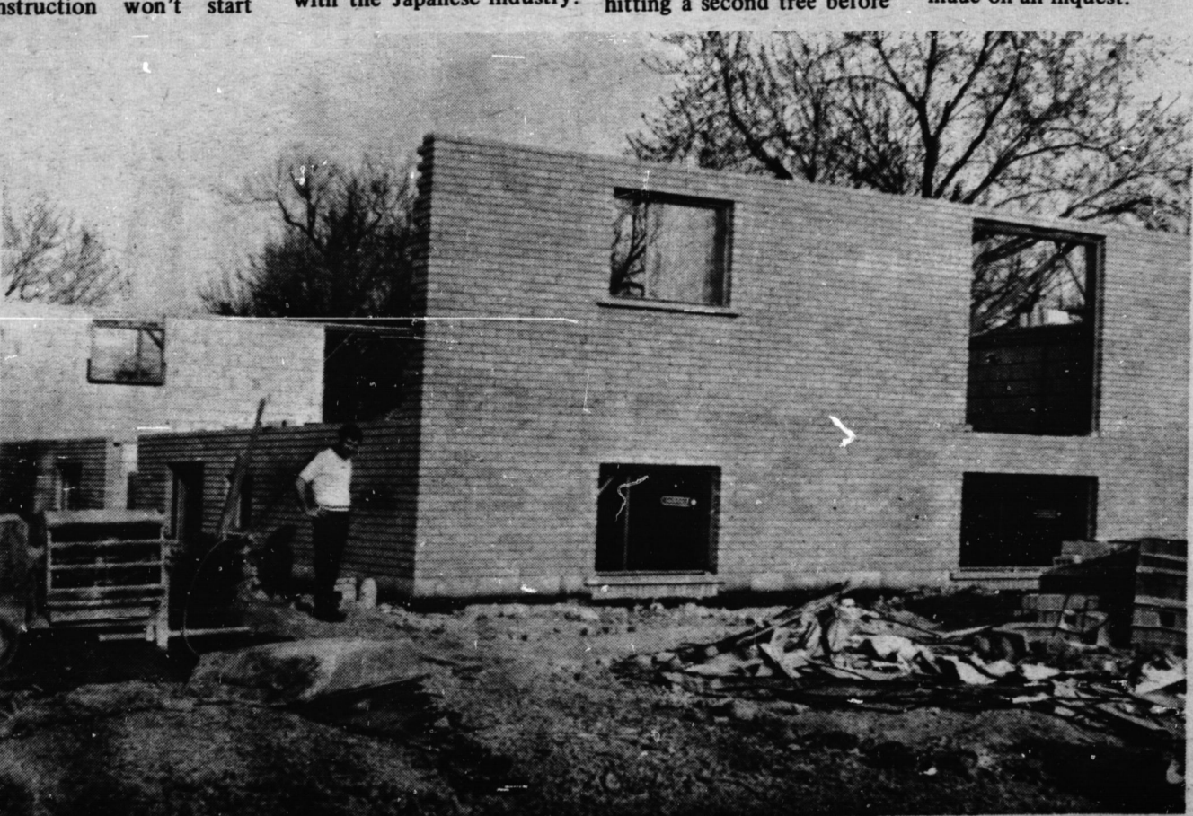
Another apartment building is being constructed in Jarvis. This six unit complex is off to a good start on Dennis St. (Staff Photo)
