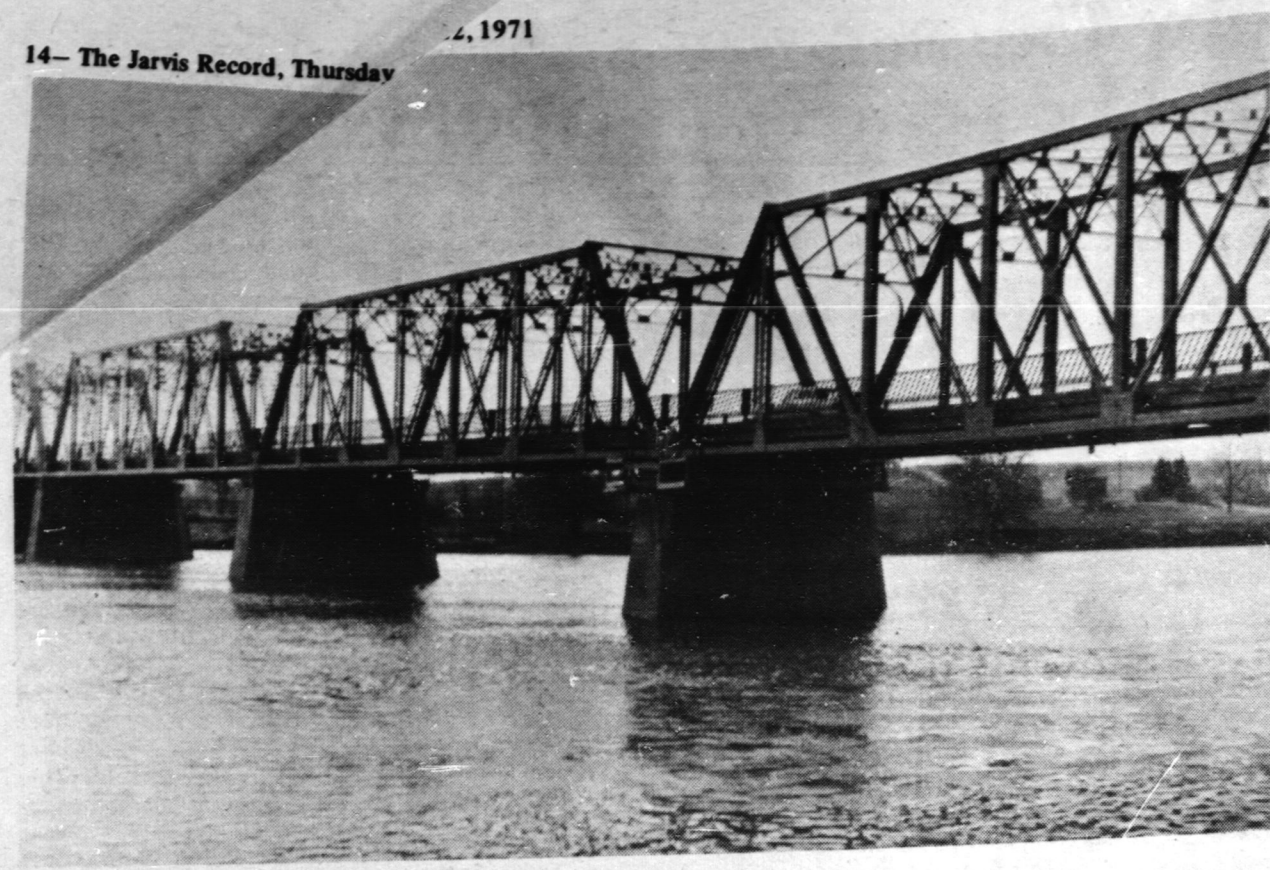
The Cayuga Bridge was opened this week for light traffic. Work crews are still repairing damage to the bridge but have got sufficiently ahead to allow single lane traffic across the bridge. A load limit of three tons has been imposed on the bridge. (Staff Photo)
