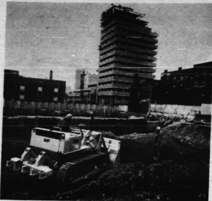
Work is progressing at the site of Canada's tallest condominium, The Fairbanks, a 42-story luxury building. Another high rise structure looms in the background, graphic evidence of progress as the Massey-Ferguson crawler speeds another project in construction being done in the Canadian capital. The city has issued building permits totaling more than $465 million in the past 17 months.
