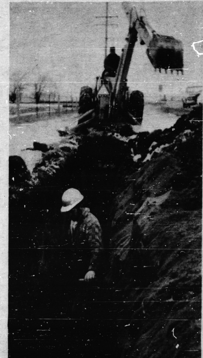
A new water main is being laid from the site of the new reservoir on the east side of the Nanticoke Road. The water will help supply the new motel under construction and a 62-lot subdivision being constructed at the rear of the hotel property. (Staff Photo)
