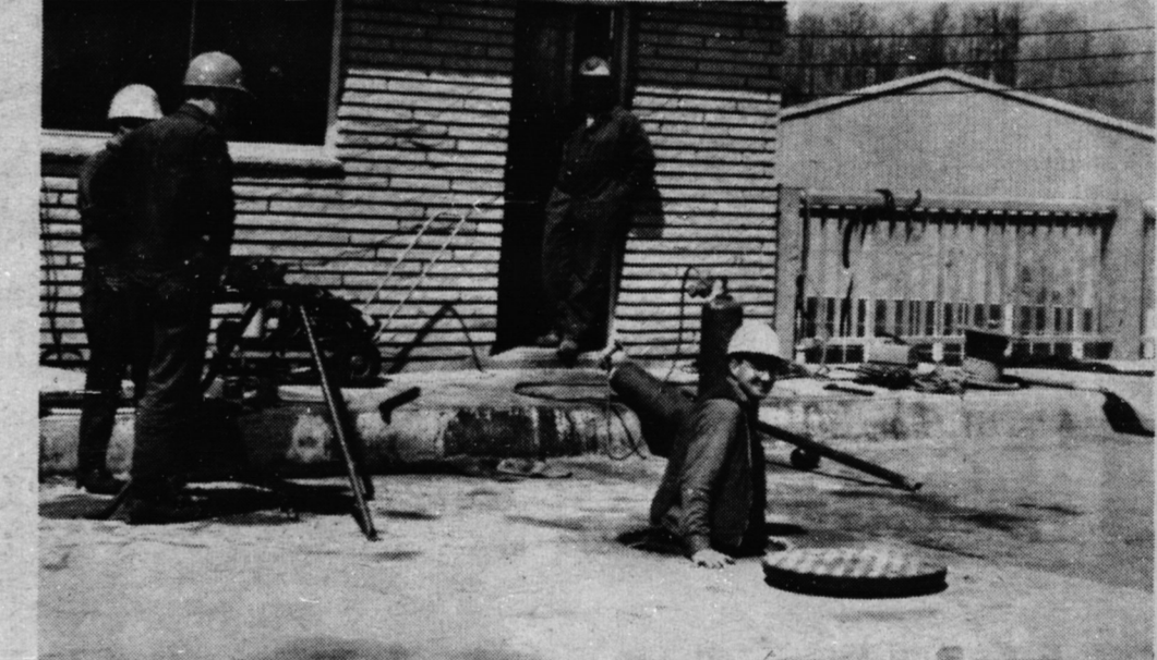
These workmen are installing new safety electrical equipment that will operate the new Port Dover lift bridge automatically. (Staff Photo)
