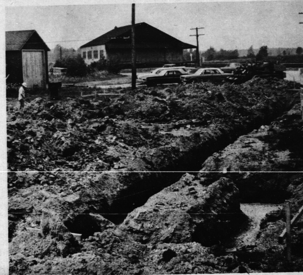
A start has been made on the building of a $37,000 general hardware store in Jarvis. Footings for the new building were poured last week, just south of the Norfolk Co-operative mill on Main St. N. The entire structure will be 90 feet long by 40 feet wide and one storey tall. (Staff Photo)
