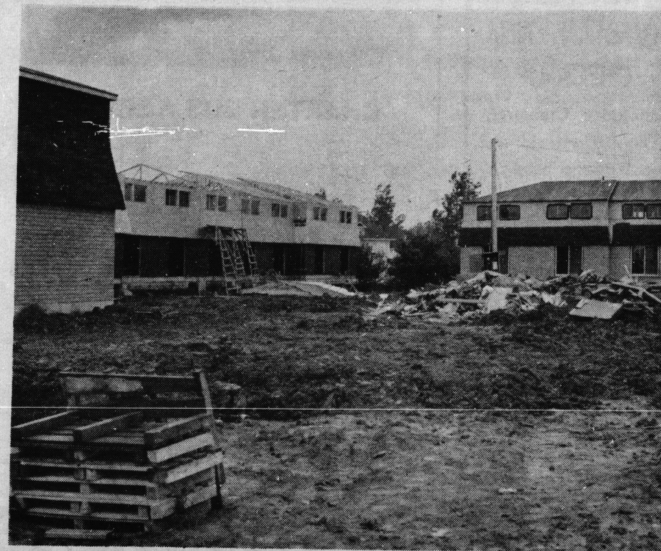
All three units of Jarvis' first townhouse complex are nearing completion with only the roof left to be completed on the middle unit. Interior work is being completed on the other two units. The townhouses are located north of Highway 3 near the Explorer Inn. Work began on the site at the end of March. (Staff Photo)
