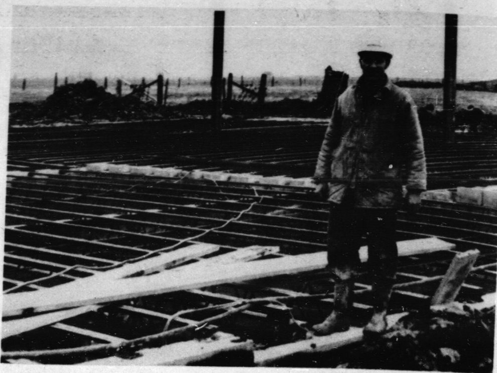
Phil Muys, superintendent of Demik Construction is pictured here in front of the Explorer Inn's future banquet area. Workers are presently putting up the structured steel for the first floor. (Staff Photo).
